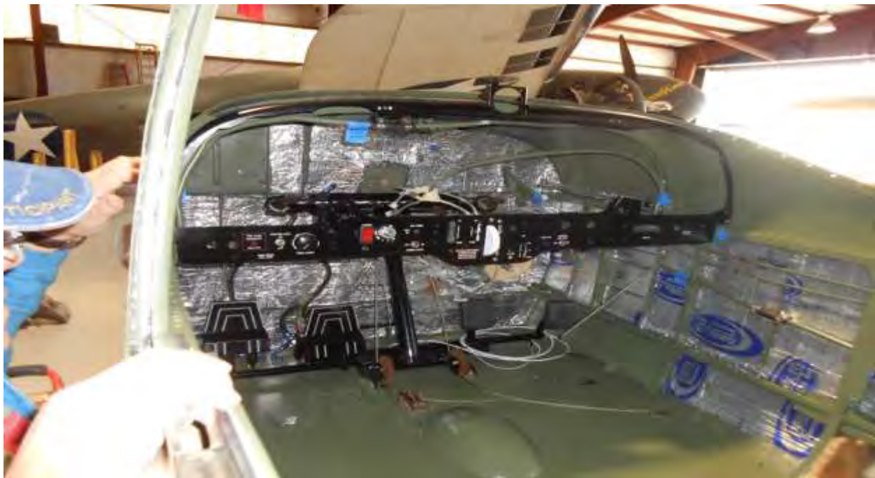
Instrument panel frame installed
